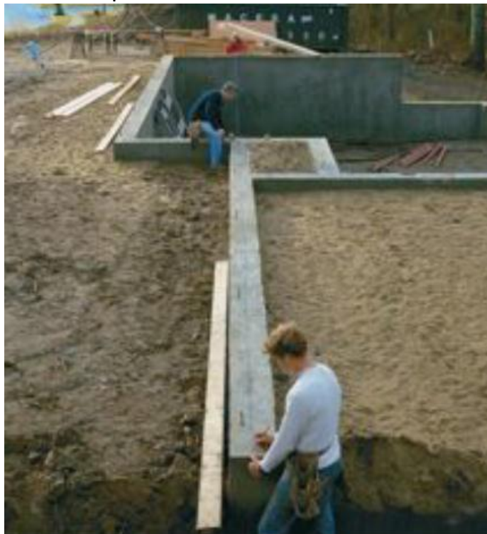
Snap chalkline to lay out the sill. The line shows where the sill's inside edge rests. If the foundation isn't perfectly square, adjust the line's position so that the sills will be. [Photo by Roe A. Osborn, courtesy Fine Homebuilding magazine © The Taunton Press, Inc.]
